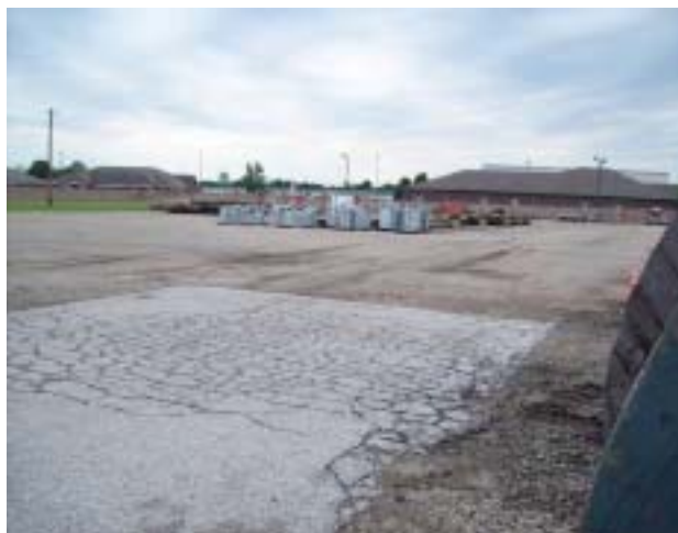
Pavement failure due to age and neglect
