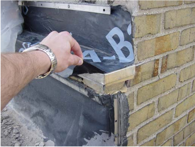
Installation of new flashing materials at the roof interface on the back sides of towers. Membrane materials require trimming for proper installation.
