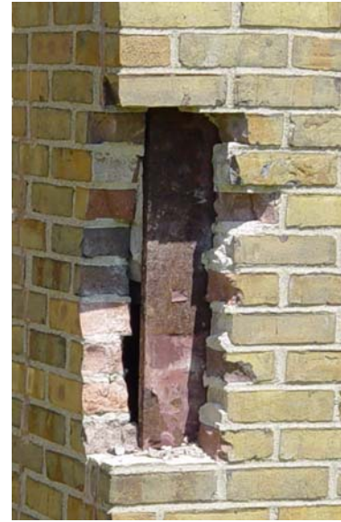
Bricks were removed at crack locations to expose rust deteriorated embedded steel columns.
