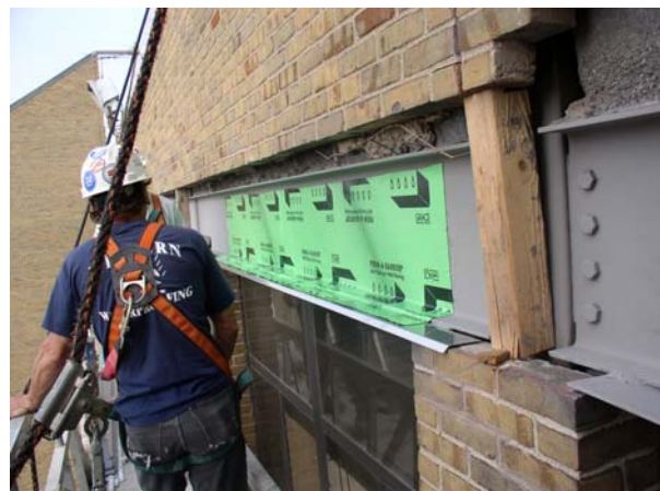
Embedded steel beams covered with two-component thru-wall flashing helped reinforce the structure.
