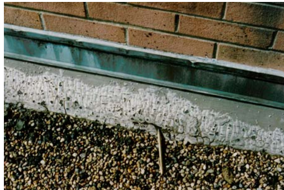
Major degradation to the existing original "paper" felt flashing along the cant juncture.
