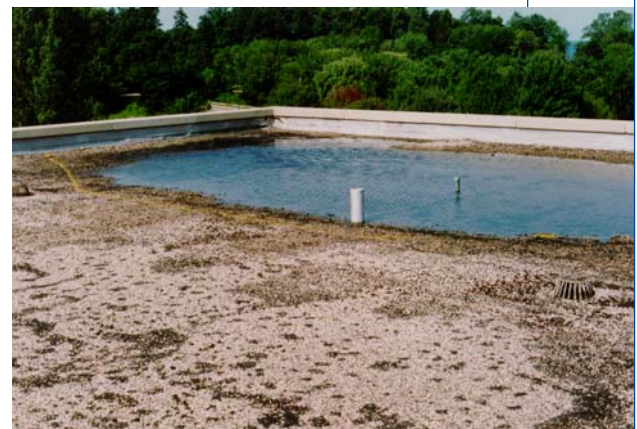
In addition to the severe ponding water conditions, the insulation is wet and saturated.
