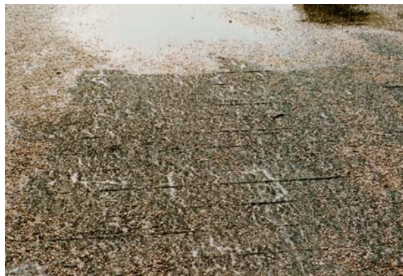
"Raised felt edges" are prevalent due to inadequate protective surfacing at this location.
