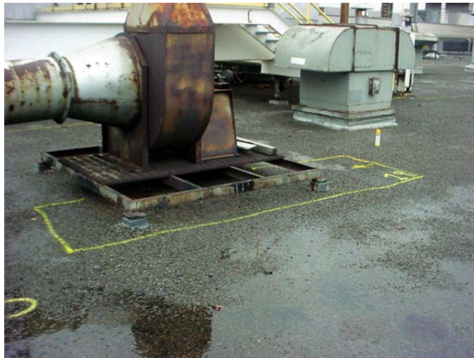
Many pieces of rooftop equipment exhibited areas of wet insulation due to inadequate flashings and extensive rooftop traffic.
