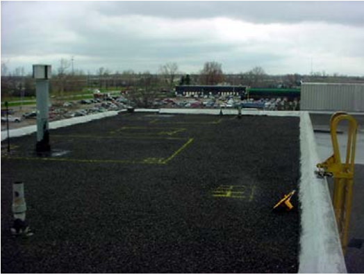
Approximately two million dollars of reconstruction occurred in areas exhibiting extreme degradation and wet insulation.
