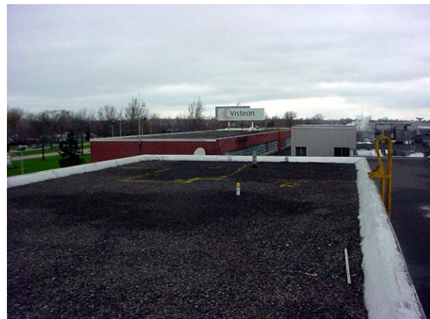
Areas of wet insulation were delineated on the roof using paint and were also denoted on detailed roof schematics.
