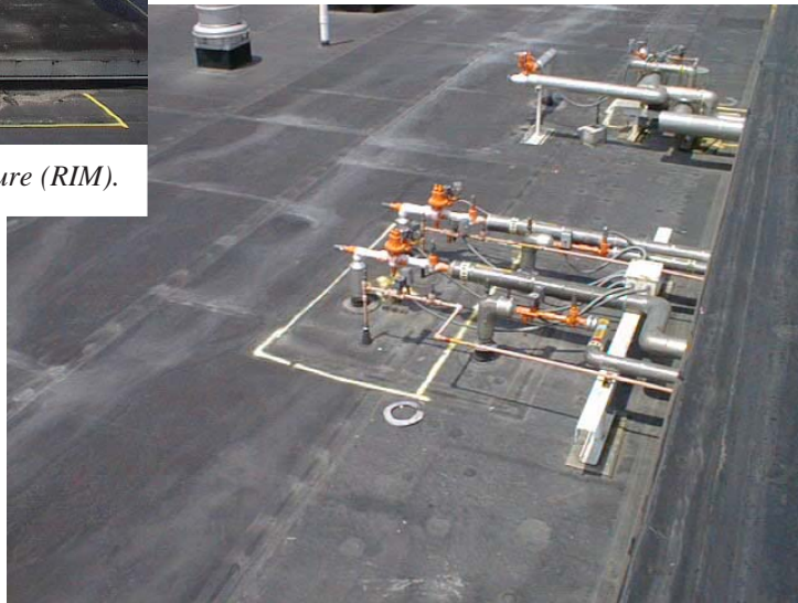
Roof top equipment has penetrated the roof membrane and caused wet and saturated insulation.
