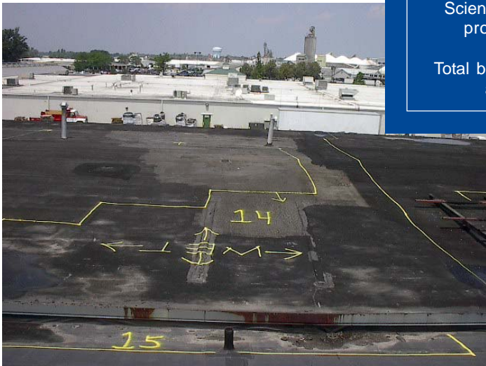
Field of roof displays Random Intermittent Moisture (RIM).
