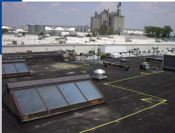
Wet area comprised 6,608 sq. ft. and encompassed the entire perimeter of this roof area.
