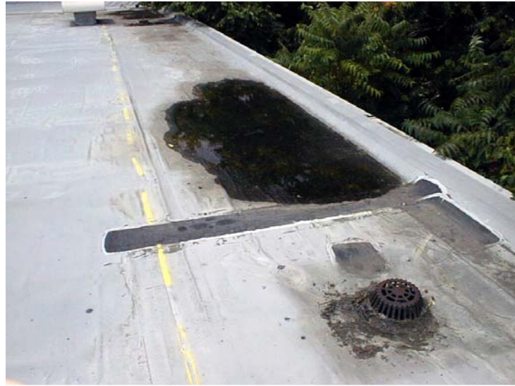
Splits and fractures in the membrane had been repaired previously without removing wet insulation beneath.
