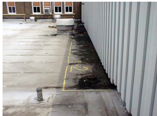
Areas of the roof with wet insulation were later repaired to extend the roof service life.
