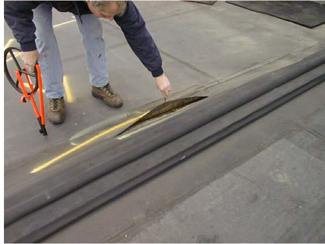
Flashing lap is open and leaking at the expansion joint.
