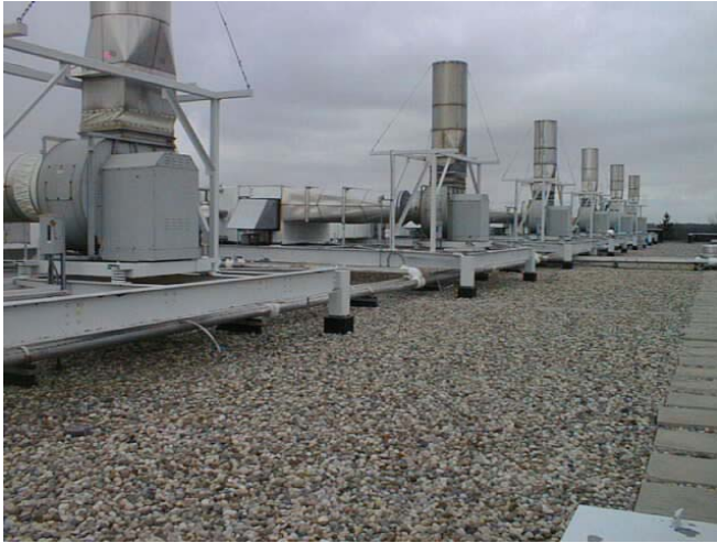
Overview of Joint Laboratory rooftop equipment and projections
