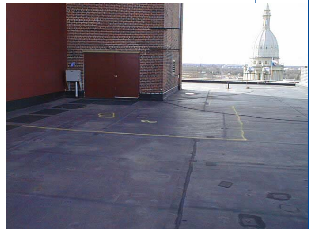
The StructureScan™ Survey revealed wet, saturated insulation at this location. Deficiencies in the flashings appear to have allowed this moisture ingress.
