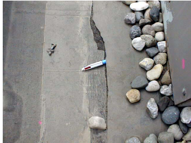
Open membrane laps were observed at various locations.
