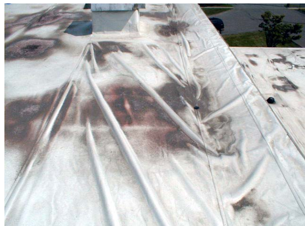
An existing roof was retrofitted with a new Durolast membrane. This roof shows deficiencies at the perimeter and wrinkles in the membrane.
