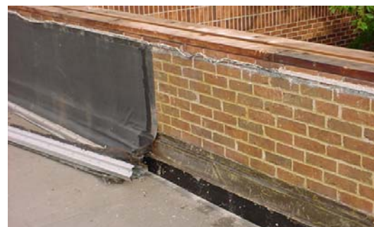
Severe leakage had occurred in the original roof system.
