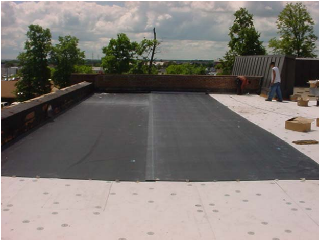
Field Quality Assurance was an important part of the construction process - ensuring a quality end product.
