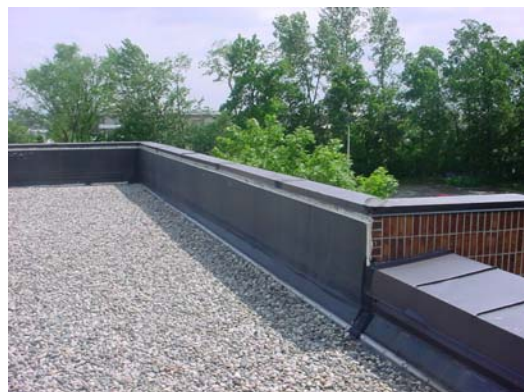
The original roof was experiencing severe leakage and had a premature service life due to lack of detail in the design.
