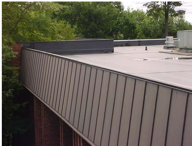
The new roof was constructed with careful attention to detail to prevent the premature failure which had occurred on the original roof.
