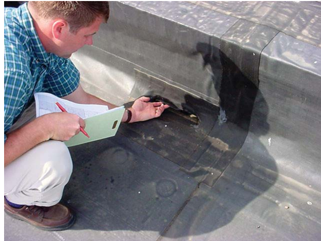
Previous repairs were inadequate and allowed moisture into the roof system.
