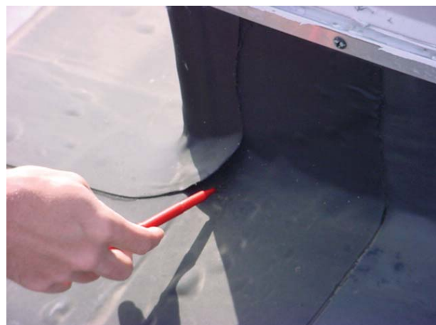
Open seams were evident at perimeter flashings.
