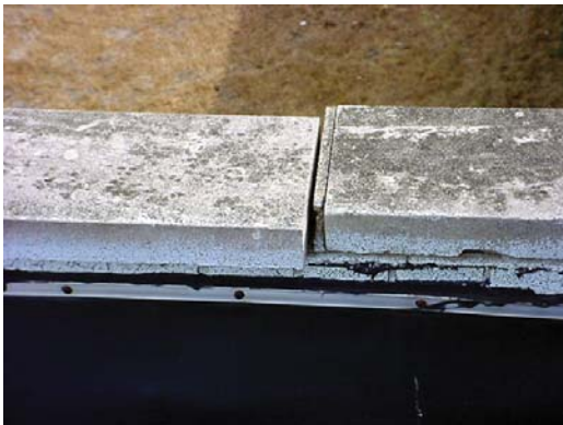
Coping stones were degraded and no longer providing protection for the parapets.
