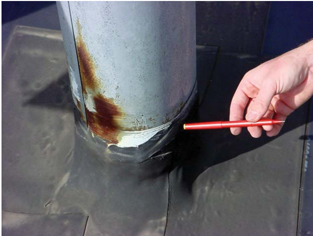
Penetrations were inadequately flashed and were showing signs of leakage.
