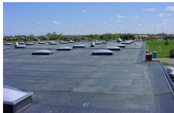
Areas of the roof included a number of skylights which required special attention and detailing.
