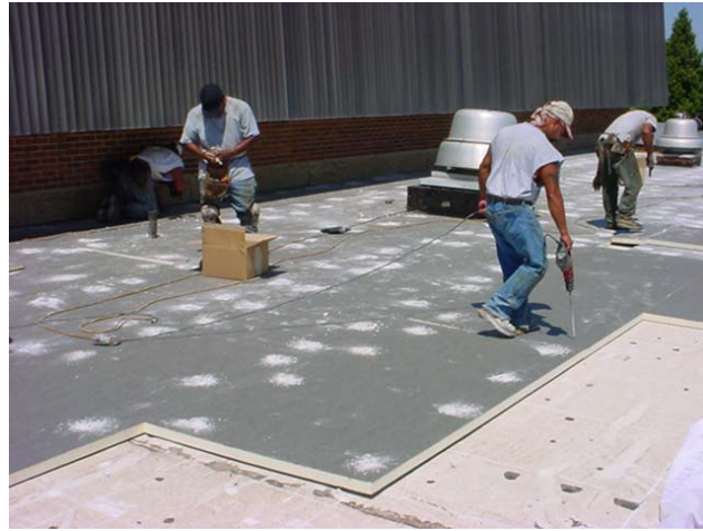
The insulation boards for the replacement roofs were mechanically attached to the deck.
