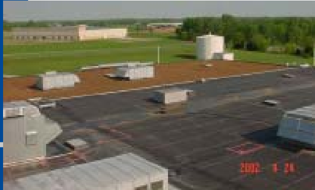
Overview of wet insulation markings and field of the roof.
