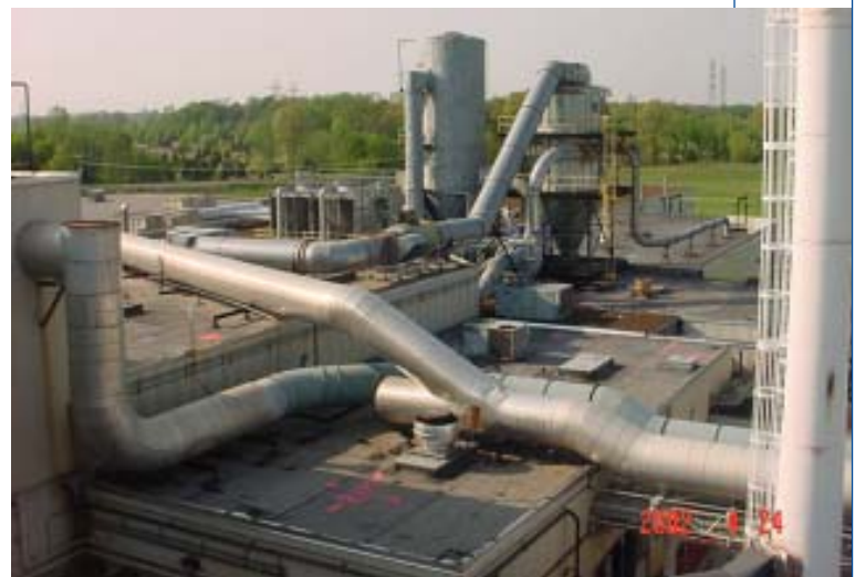
Extensive rooftop equipment is required for the manufacturing process.
