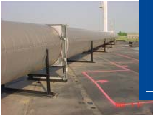
Overview of extensive ductwork resting on the roof surface.
