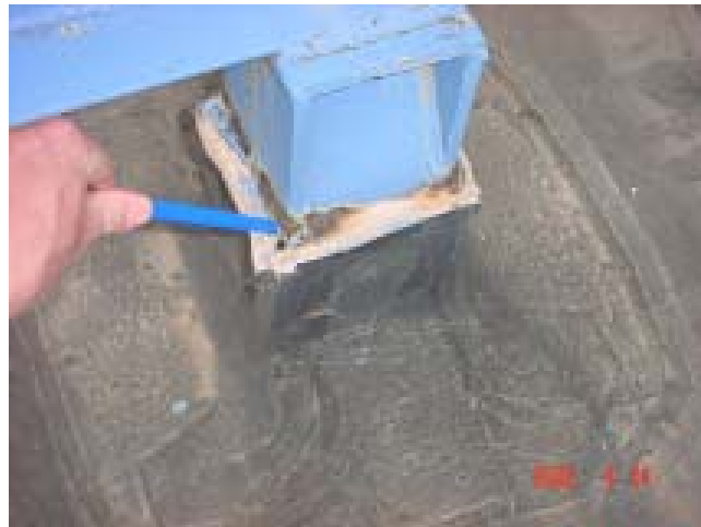
Roof equipment is not properly flashed. Previous caulking repair was unsuccessful.
