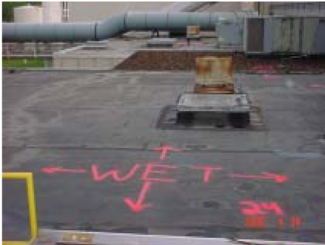
Areas of wet insulation were detected by the infrared StructureScan™ Survey.
