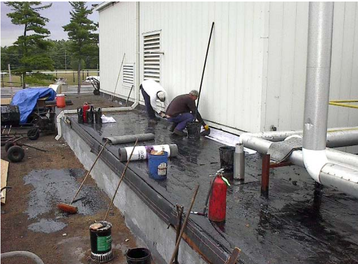
The contractor worked double shifts in order to meet Parkedale Pharmaceutical's deadline.
