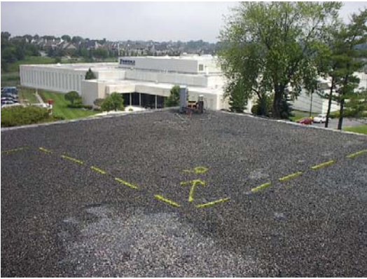
The StructureScan infrared thermal imagery scan revealed the areas of wet insulation during design development.
