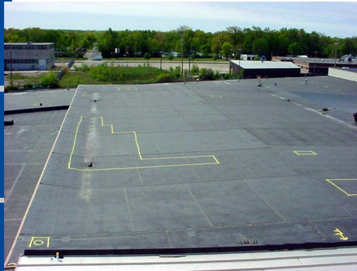
Overview of the Alma Plant. Areas of wet insulation were marked during the StructureScan Survey.
