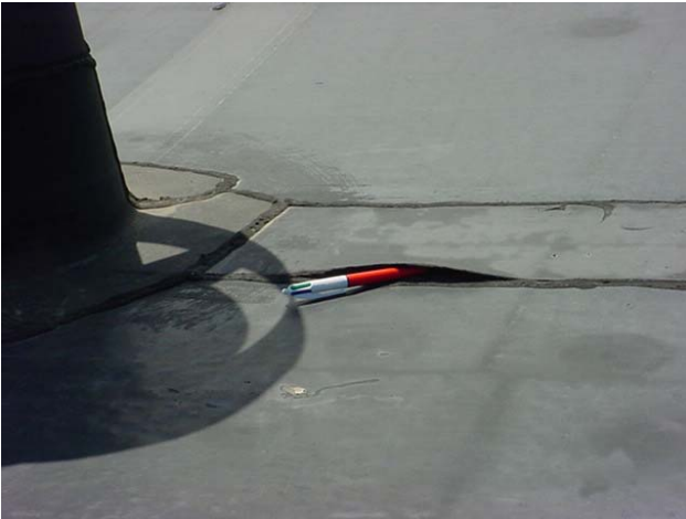
Seams, one of the weakest parts of the single-ply roof system, were no longer properly adhered and sealed.
