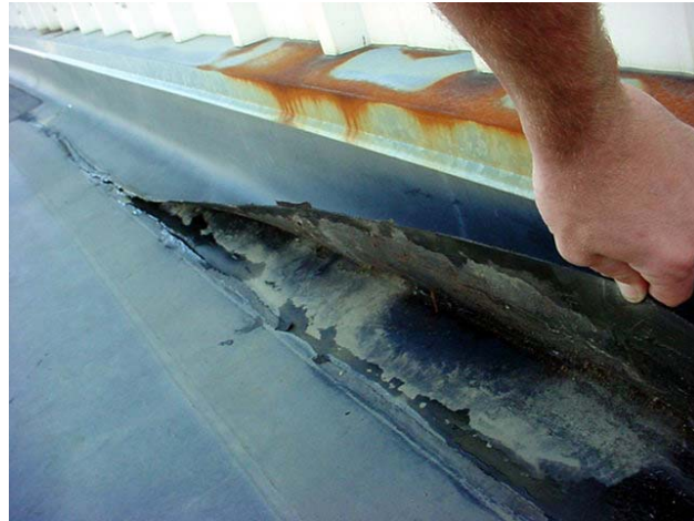
Flashings were disbonded and open at various locations, allowing moisture ingress into the roof and wall systems.
