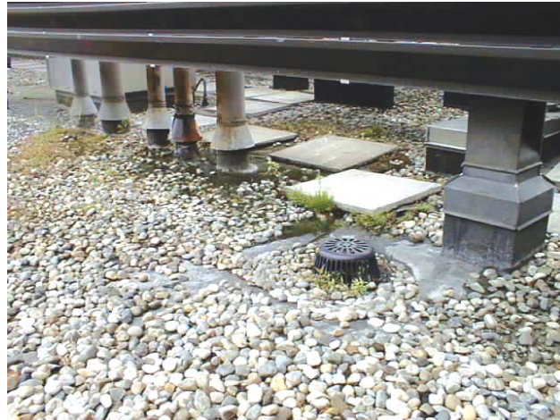
Debris has accumulated around the drain and moisture in the membrane has allowed vegetation to grow on roof surface.
