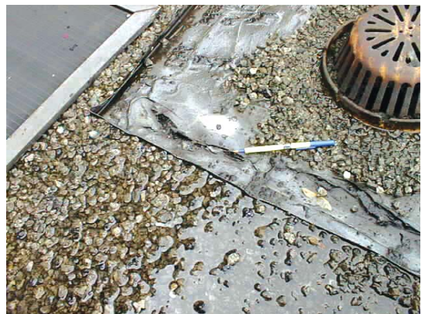
Open flashing observed at roof drain.
