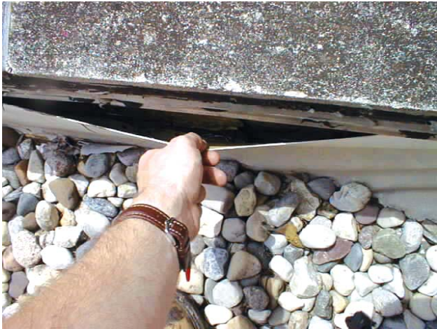
Inadequately secured flashing observed at parapet wall.
