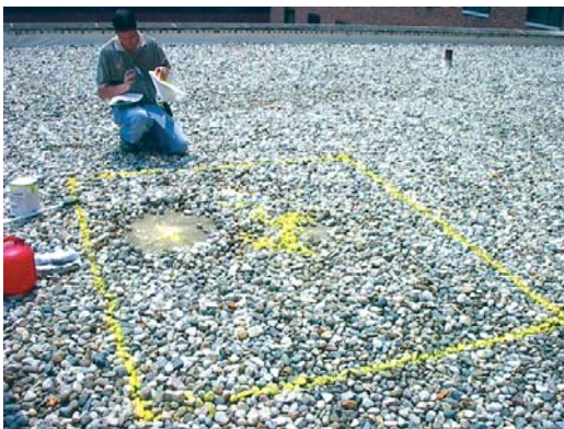
Area of wet insulation identified during the StructureScan survey. A test cut was performed within the area to confirm the results.
