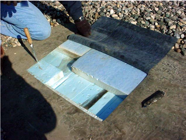
Migrating ballast caused the insulation underneath to become displaced and damaged.
