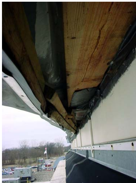
Perimeter edge nailers had come loose, migrating from the edge and causing the exterior flashing to come unfastened.
