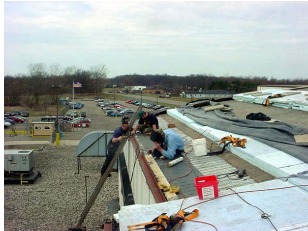
Perimeter edge details were reconstructed with adequate structural integrity to support the weight load of the roof.
