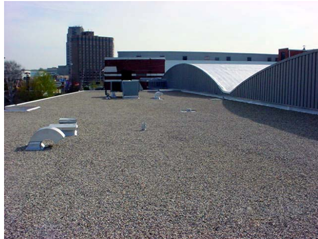
A new slip insert counterflashing and deck replacement were part of the roof replacement project. (AFTER)
