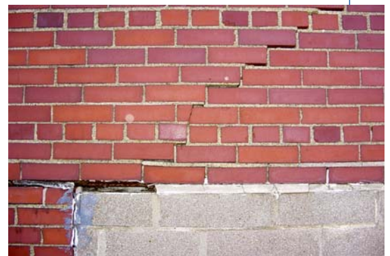
The masonry wall was exhibiting significant distress and required structural remediation.
