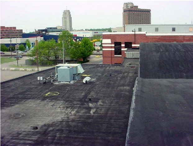
The roof was experiencing significant distress and required replacement. (BEFORE)
