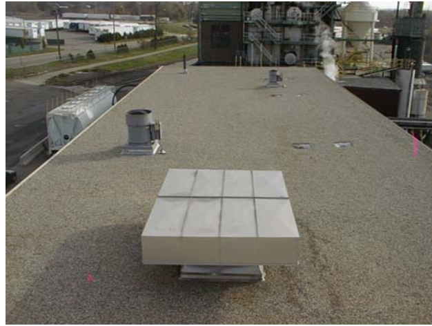
New roof assembly included built-up membrane with modified cap sheet, flood coat, and roofing aggregate.
