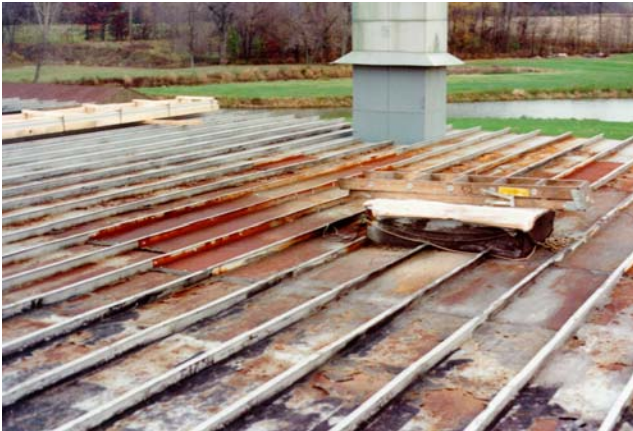
Corrosive chemicals from the plating manufacturing process were expelled from the roof top projections and resulted in massive corrosion to the existing metal roof assembly.
