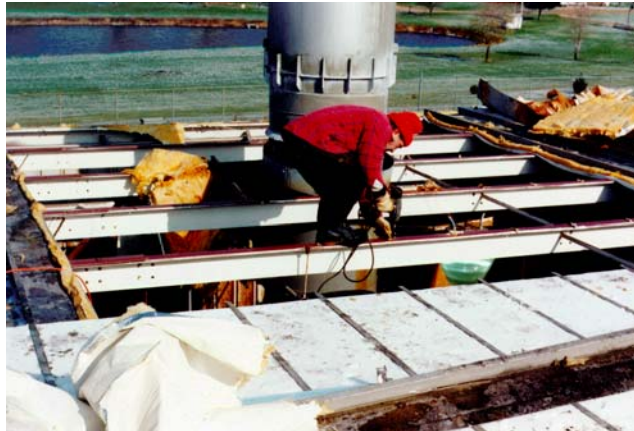
Complete removal of the existing metal roof assembly was required due to the extensive degradation of the original system.
