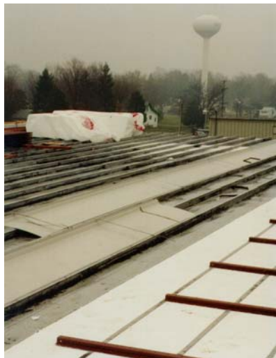
The new metal roof was installed retrofit over the existing metal roof.
