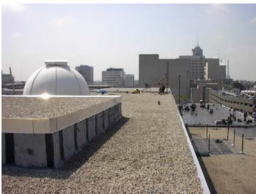
Extensive detailing was performed to ensure that all the special elements of the roof were properly flashed, ensuring watertight integrity.
