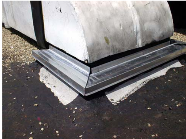
Tapered insulation, crickets, and saddles were installed, particularly around projections, to provide water dispersion.
