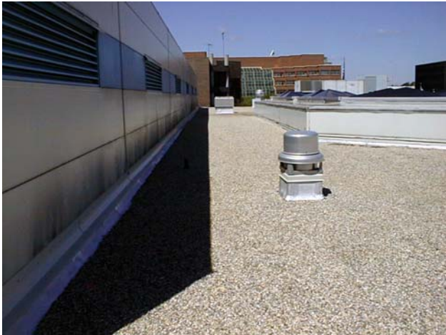
A new tie-in was designed along the wall transition to accommodate movement and maintain watertight integrity.
