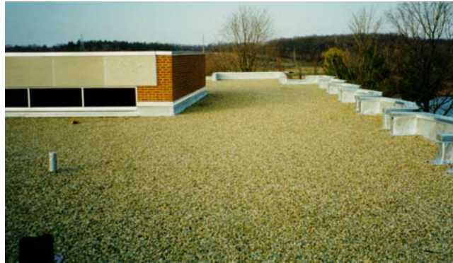
The new built-up roof system, which incorporated zoned insulation, replaced the original roof.
