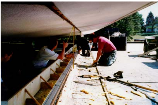
Original flashing heights around window panels were of inadequate height for watertight integrity.
