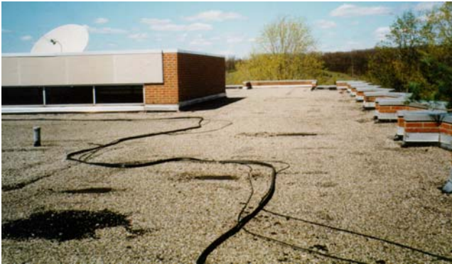
Existing roof was extremely degraded, experiencing leakage, and at the end of its service life.
