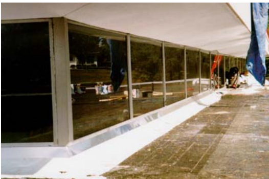
New flashing details and window panels were installed as a part of the roof replacement.
