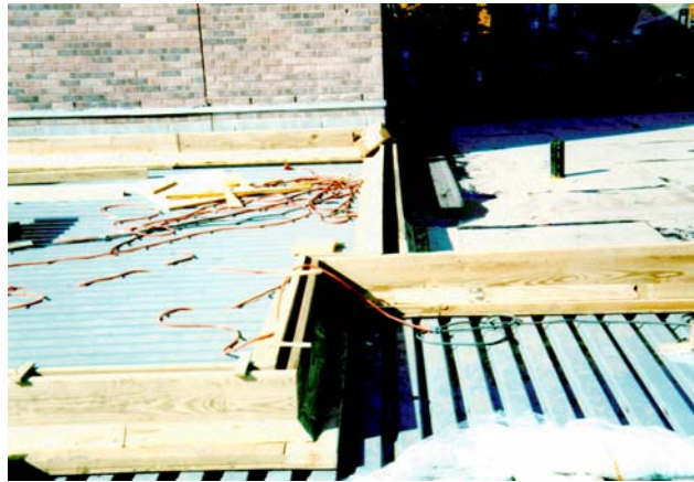
Repairs were made to the existing metal deck before installing the new roof system. New lumber curbing was installed to raise the height and allow for new expansion joint and coping covers.
