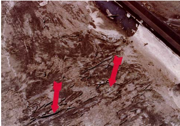
Previous roof had bare exposed felt which allowed "wicking" of moisture into the roof system..
