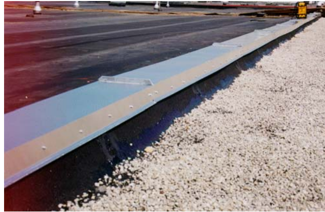
Attention to detail is evident in the expansion joint flashing and sheet metal coping.
