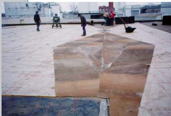
Saddles were designed as a part of the new roof system in order to help eliminate ponding water.
