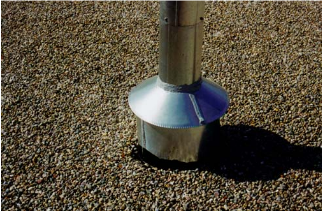
Rooftop projection is properly flashed with a stainless steel sleeve and a rain collar.
