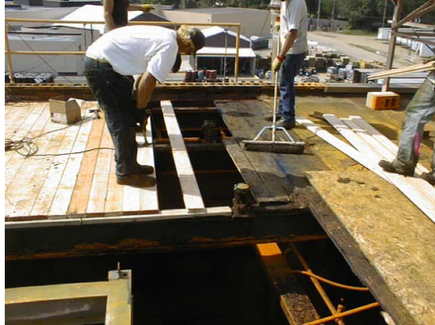
New decking was installed to provide structural integrity for the roof and the rooftop equipment.
