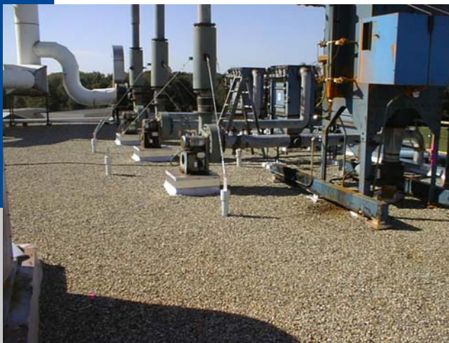
Extensive rooftop equipment and penetrations received careful attention to detail as flashings were incorporated into the roof replacement project.
