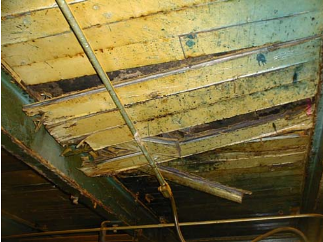
Existing wooden deck was completely degraded due to the extensive, prolonged moisture ingress in the roof system.
