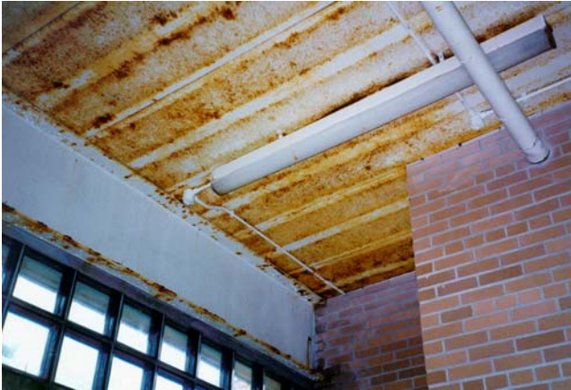
Metal roof deck is extremely rusted and degraded, requiring replacement. Structural steel beams have surface rust and lead-containing paint, requiring restoration.
