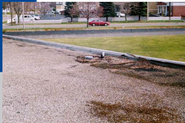
Extreme degradation, including vegetation, is evident on existing roof system.
