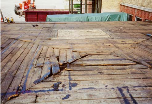
Deteriorated wood decking was not structurally sound.
