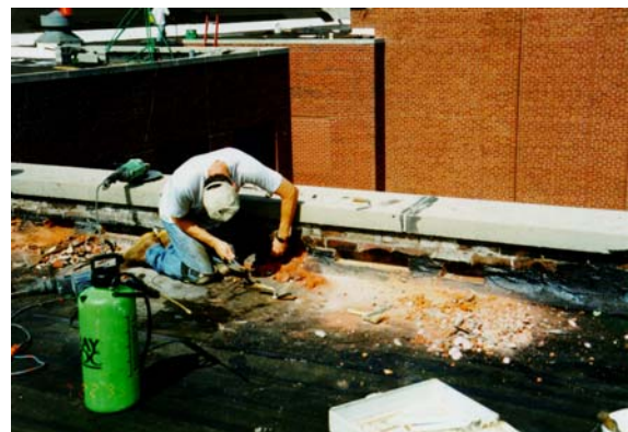
Cracked or fractured masonry units were replaced as a part of the restoration process.
