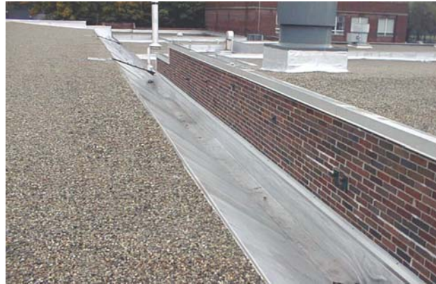
StructureTec conducted Field Quality Assurance to ensure that all the details of the project were correct.
