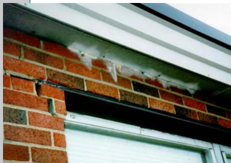
Window lintel and masonry degradation. Also, previous unsuccessful caulking.
