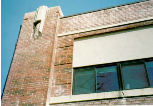
Masonry mortar joints were deficient. Concrete belt stone was cracking and spalling.
