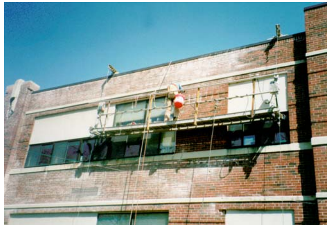
Deficient mortar joints were saw-cut to remove existing sealant and then tuckpointed with new mortar.
