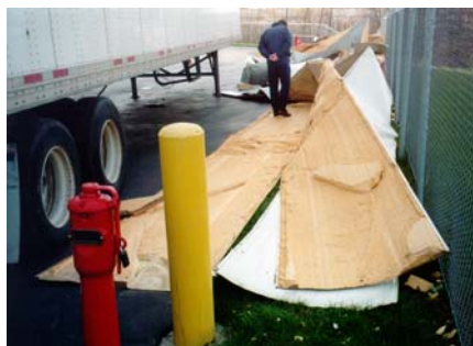
Twelve panels blew off the tower, landing in the nearby parking lot.
