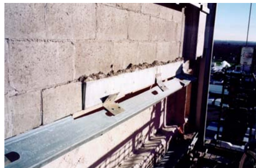
A deficient subframing system was one of the primary causes of the blow off.
