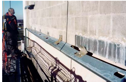
Extensive observation and analysis was performed on the existing construction to determine the cause of the failure.
