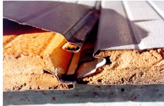
Exterior cladding consisted of sandwich panels with an outer metal skin and insulation in the middle.
