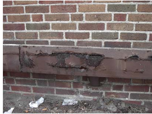
Rust and corrosion evident on steel guardrail along the base of wall.
