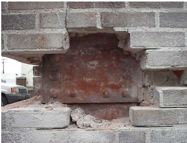
Wall opening allows embedded steel flange and splice plate to be observed.
