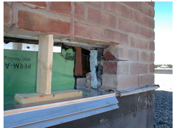
New through-wall flashings consisting of stainless steel and a flexible waterproofing membrane were installed at upper wall levels.
