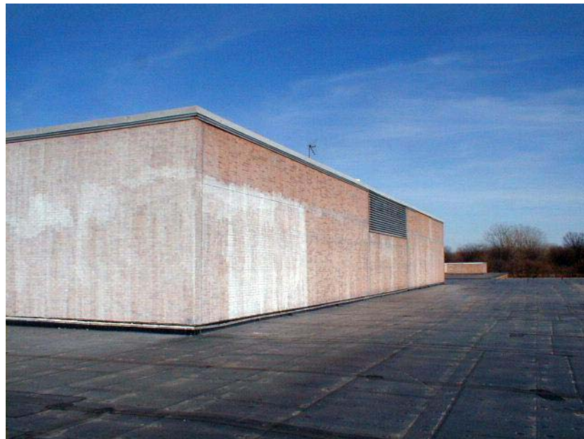
Residue staining was more severe on several areas of the walls.
