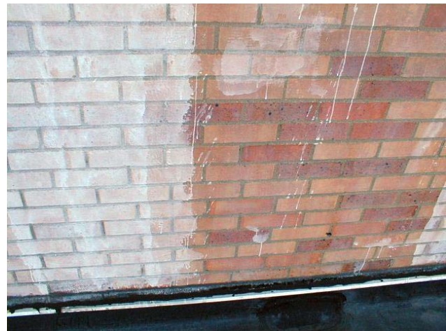
Methods, means, and procedures for removing the residue were tested on strips to determine effectiveness.
