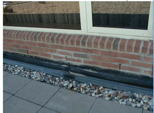
Water ingress caused by masonry distress and deficient through-wall flashings.
