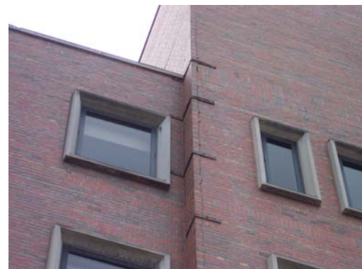
Overview of the larger crack and extended steel straps at the upper portion of the wall.
