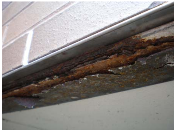
Corroded lintels observed and detected during a StructureScan TM survey
