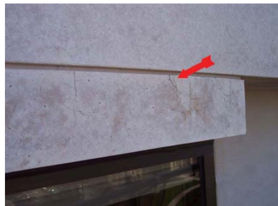
Crack in precast concrete panel allowing water infiltration
