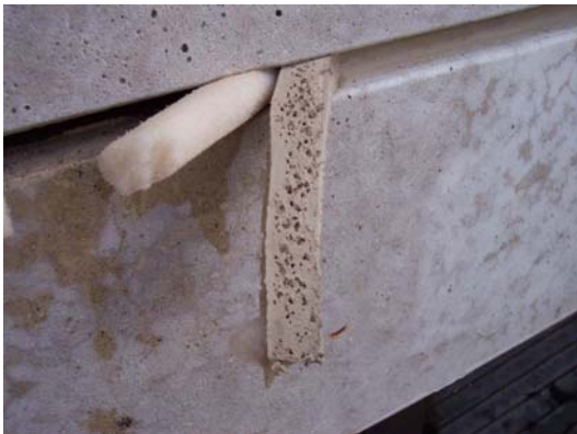
Voids in joint sealant between precast pane causing premature failure and openings
