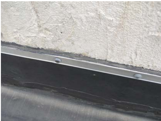
Failed sealant along top of roof flashing termination bar allowing water infiltration (Inadequate design and construction of original flashings)
