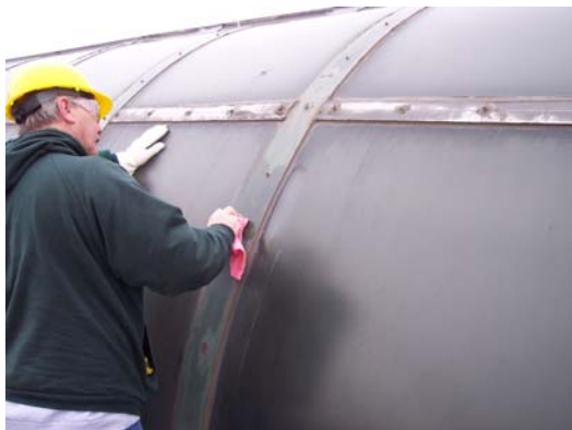
Surface preparation was a critical factor in the success of the installation
