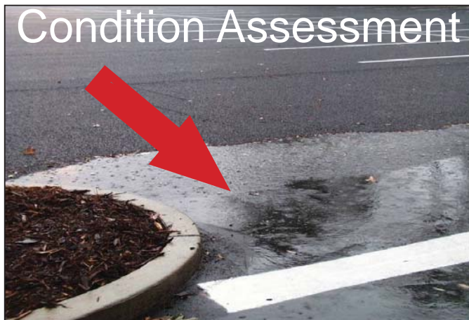
Improper drainage causing ponding water
