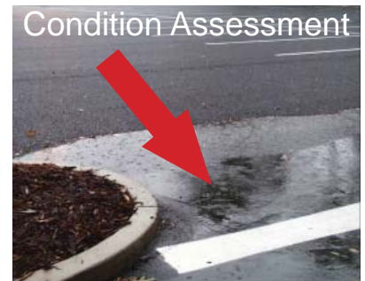
Improper drainage causing ponding water
