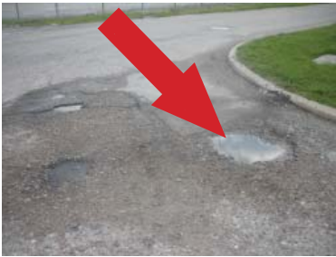
Surface deterioration - potholes and severe cracking
