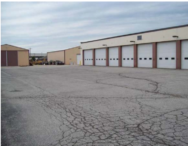
Pavement failure due to age and neglect.
