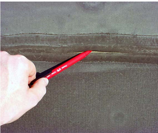
The lap sealant at the membrane seam is deficient in locations.
