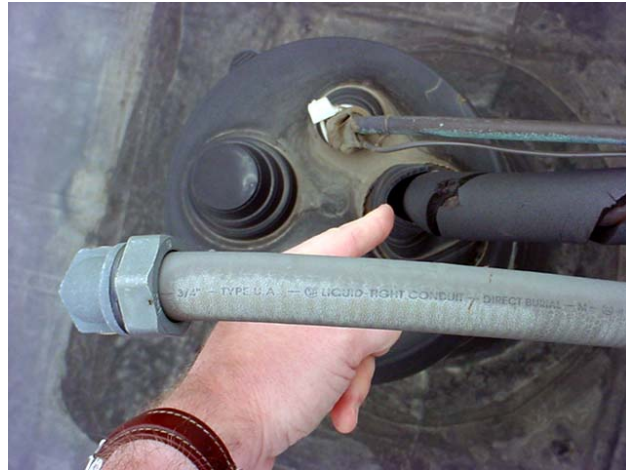
The top of this pipe projection is no longer watertight and is a source of leakage into the building.
