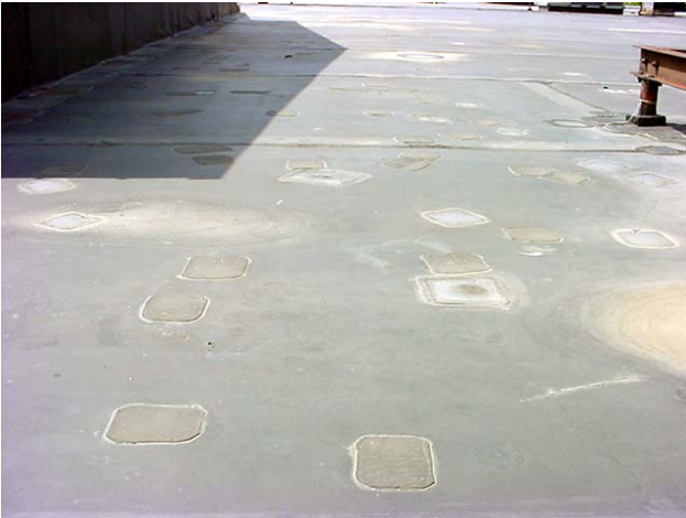
A large number of repairs were made to the roof membrane in this location.
