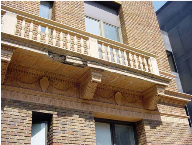
The terra cotta balcony was experiencing expansive deterioration with vertical cracking of spindles and spalling of the underside.
