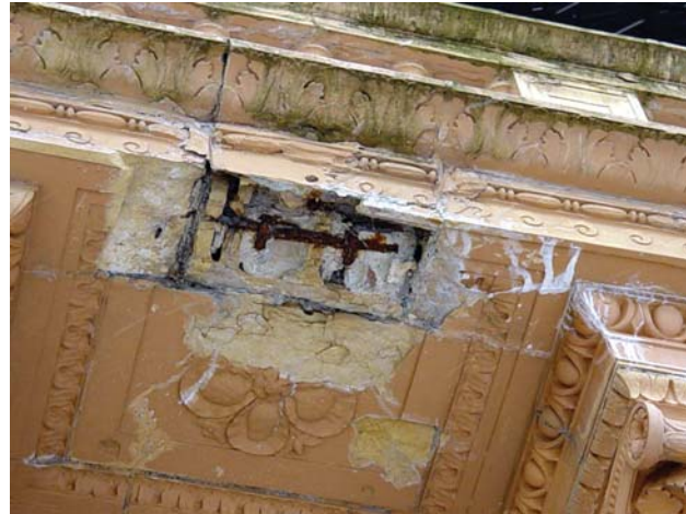
The spalling of the terra cotta on the balcony was caused by the rusting of the embedded steel, as well as extensive freeze/thaw cycles.
