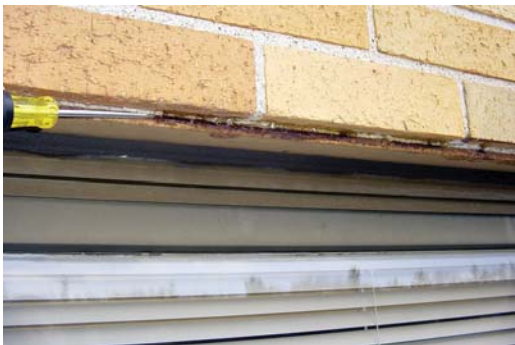
The embedded steel shelf angle is exhibiting rust deterioration indicative of failed coating and a high concentration of moisture.
