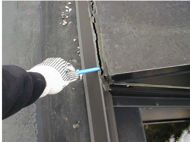
Deteriorated sealant is evident at these wall panels.
