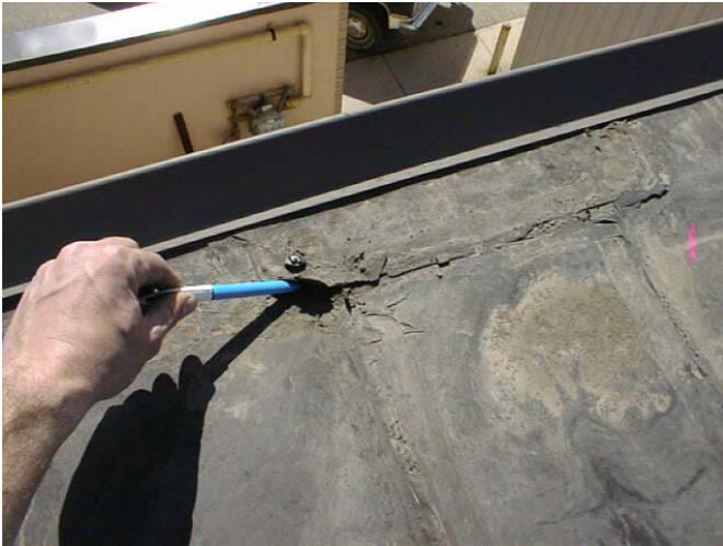
Open lap observed at the perimeter edge of the roof membrane.
