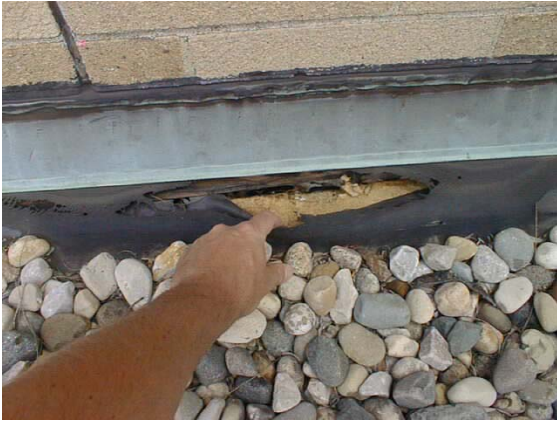
Deteriorated membrane observed at wall flashing. Exposed wood nailer and insulation observed.
