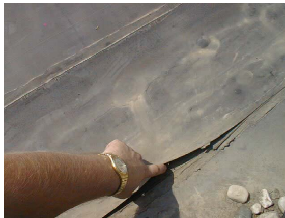
Open lap observed. EPDM seams appeared to be deficient.
