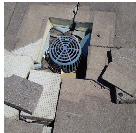
Damaged protective board around roof top drain. (Protected Membrane Assembly)
