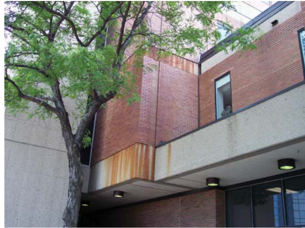
Heavy rust staining is evident on the concrete. The mortar is deteriorated, and vegetation is growing too close to wall.
