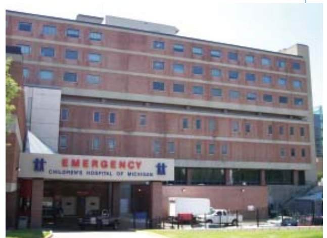
Periodic staining on exterior masonry.
