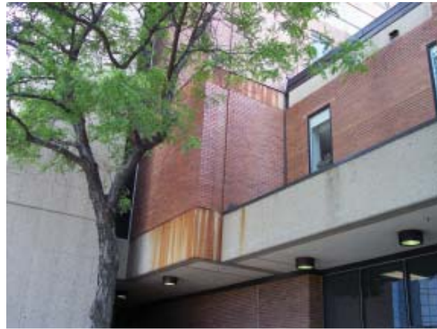
Heavy rust staining is evident on the concrete. The mortar is deteriorated, and vegetation is growing too close to wall.
