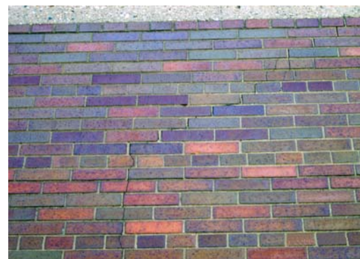
Multicourse, stair-step crack ran through the masonry and mortar.
