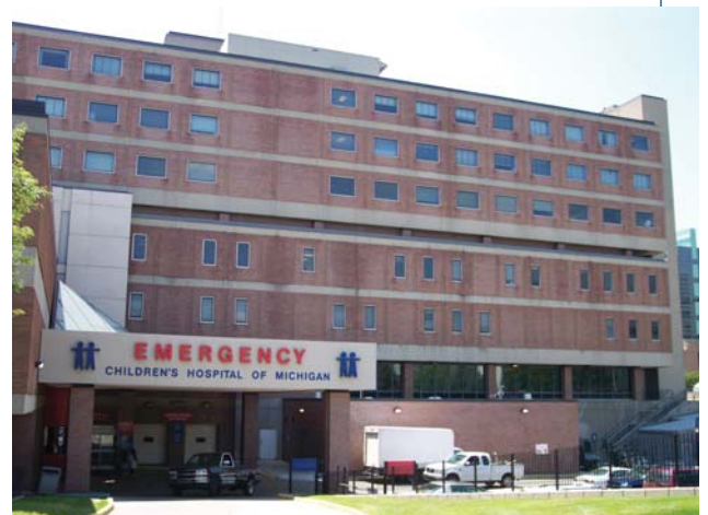
Periodic staining on exterior masonry.
