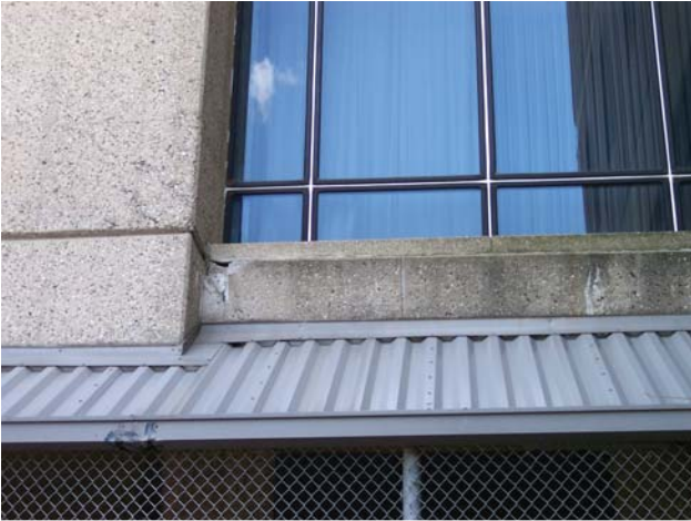
Concrete had deteriorated over time, spalling and requiring patching.
