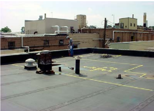
An infrared StructureScan survey was performed to determine areas of wet insulation.
