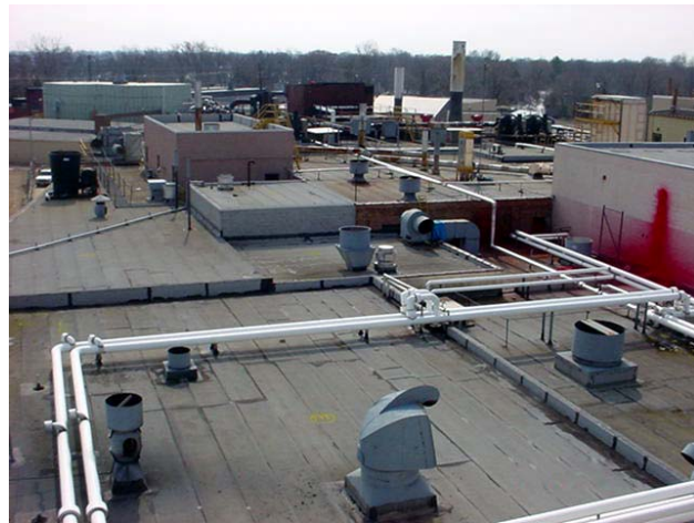
Massive square footage and extensive rooftop equipment posed a challenge during the evaluation.
