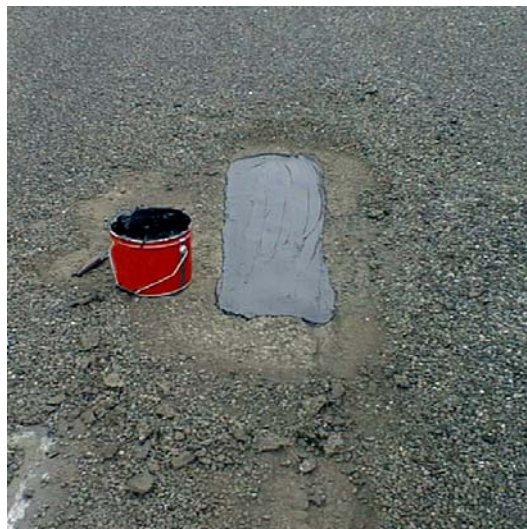
Proper methods, means, procedures, and materials were used to provide long-term repair and reinforcement of the membrane.
