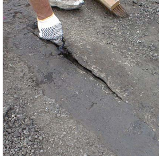
Splits in the built-up roof membrane were marked and designated for repair.
