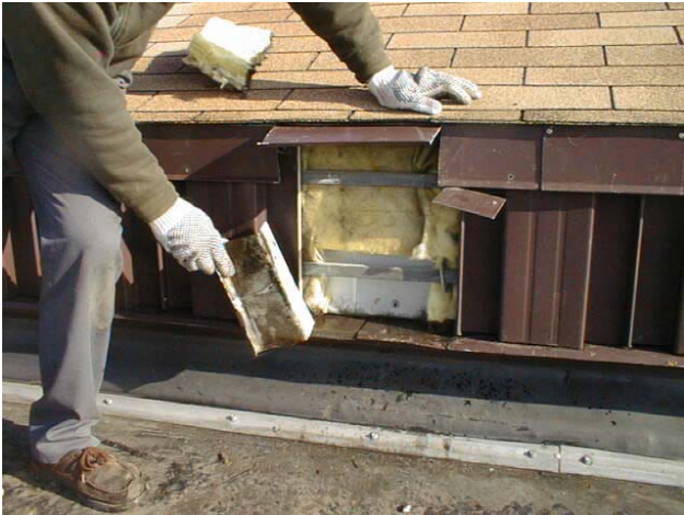
Architectural metal cladding exhibited leakage at intermittent locations.
